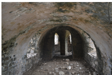
Fig. 12 Looking down the length of the basement under the access ramp to the mill above, with the distant central pillar supporting the working floor of the Diamond Keturah windmill
