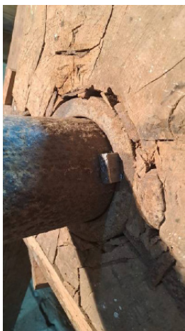
The offcut of the key protruding slightly at the front.
