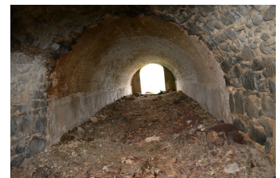
Fig. 13 The main basement at The Sight windmill is over 5 feet high and runs the full width of the windmill
