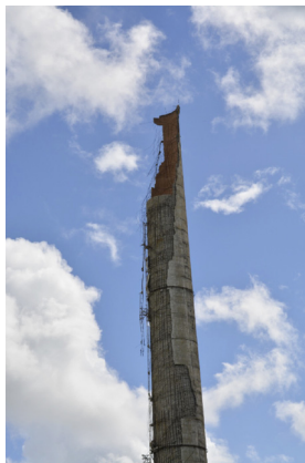
Fig. 23 Steam chimney at the former central factory at estate Bethlehem, with the western side of the reinforced concrete structure collapsing
