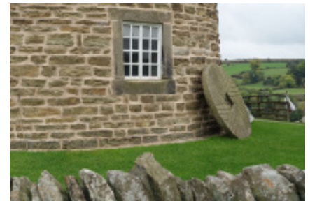
Fig. 2. A closer look at the pointing
